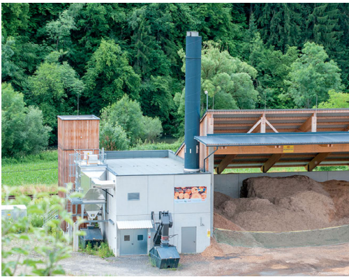
Heating plant Brückl
