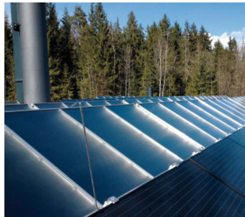
Solar thermal and photovoltaic panels on the roof of the heating plant.
