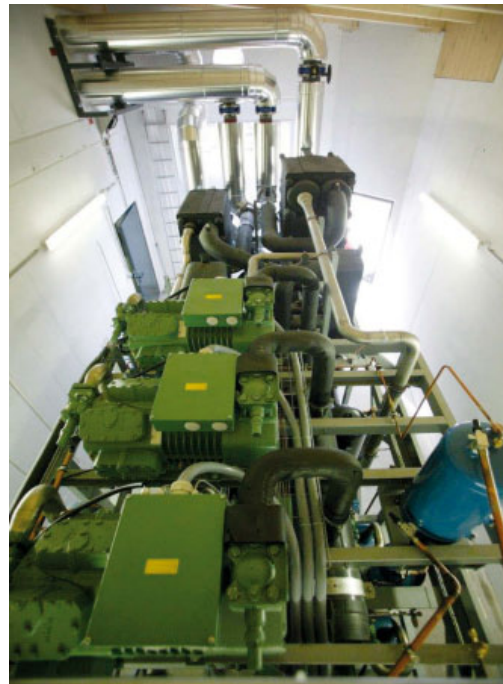
Industrial heat pump
