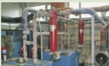
© Sattler Energie Consulting
